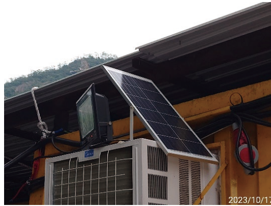
Solar-powered Lighting for Site Office
