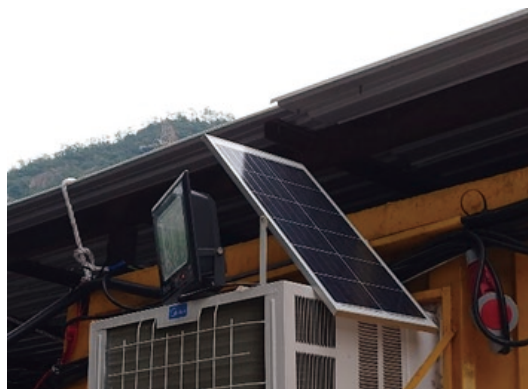
Solar-powered Lighting for Site Office
